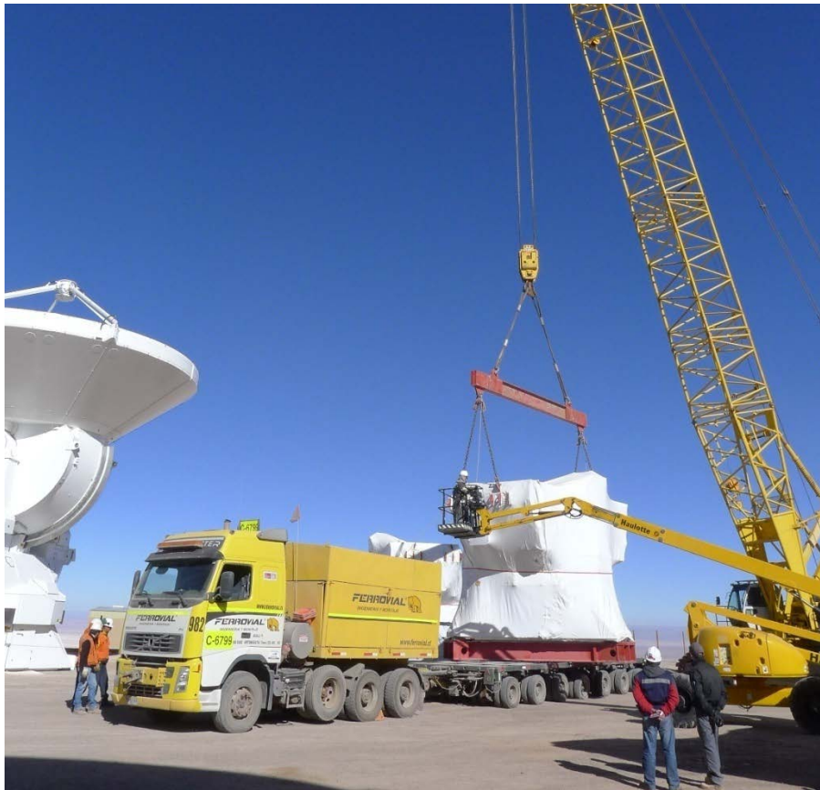
Figure 1: Unloading of the last steel structure, #25, at the OSF on September 7 th , 2012.
